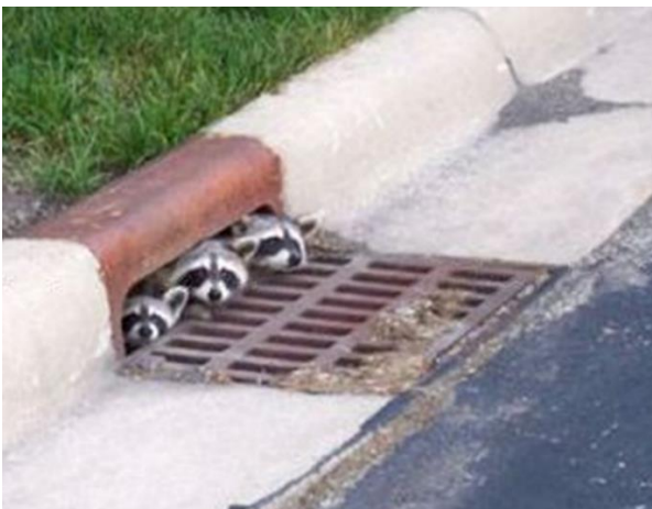
Figure 2: Typical Catch Basin Inlet
